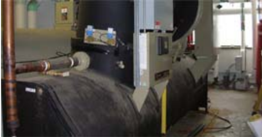
The project team installed two new 750-ton chillers to replace an antiquated 1,250-ton chiller and, more importantly, central control of distribution system components. These upgrades saved Loyola $750,000 in capital costs and $30,000 a month in energy costs.
